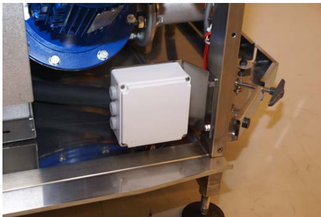
Figure 3: Detergent and rinse aid junction box
